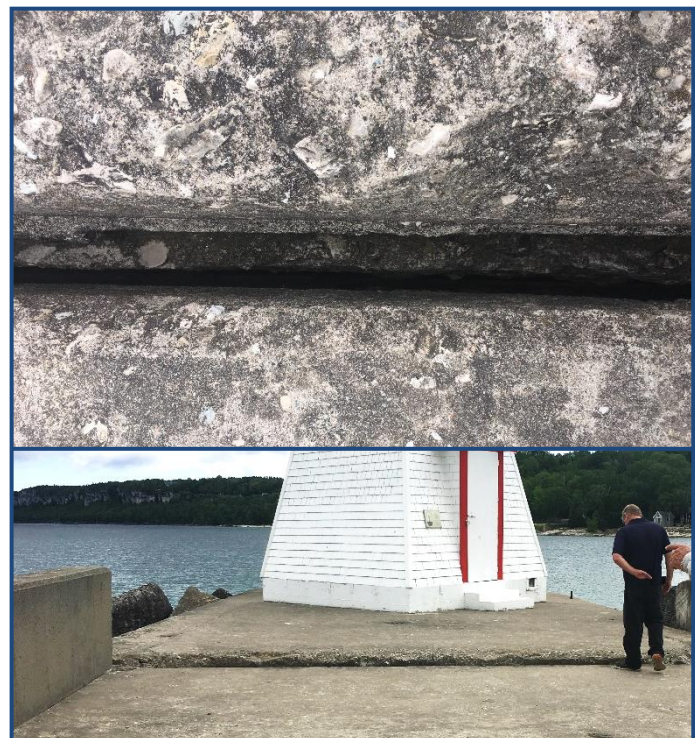
Figure 7-1: Separation of Concrete Lighthouse Base Slab from Concrete Wharf
