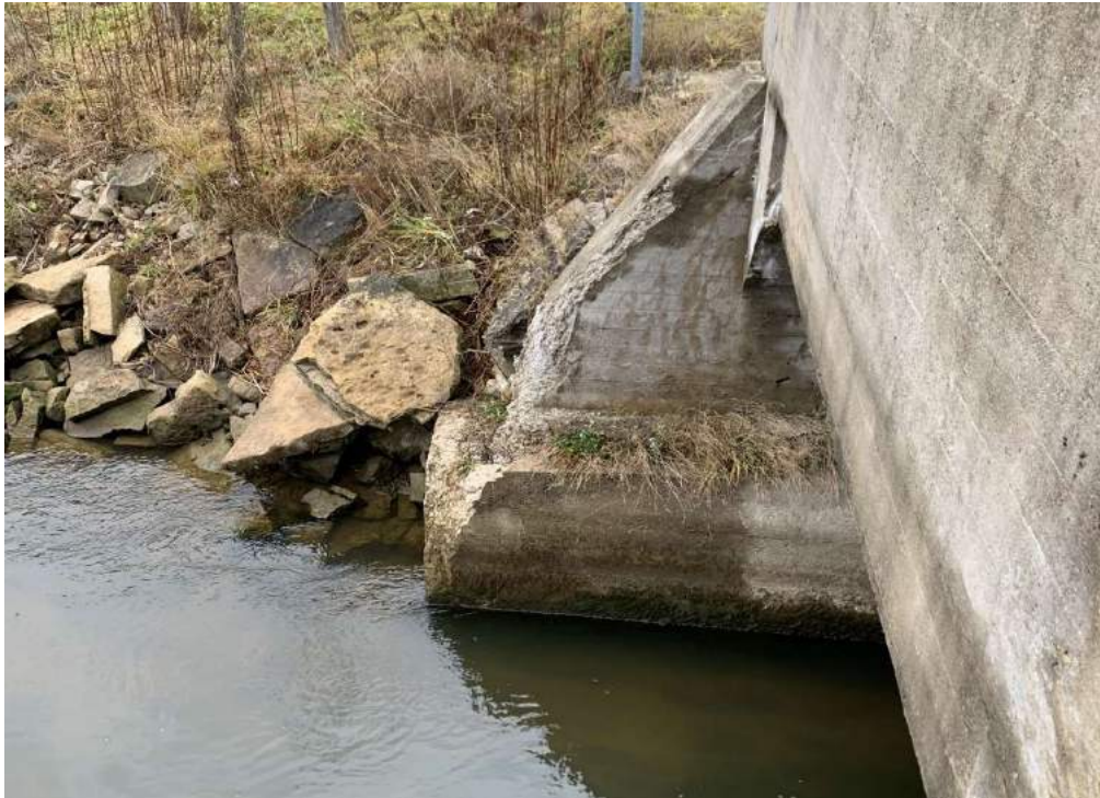
Photo 6-15: View of abutment wall and footing spalling.
