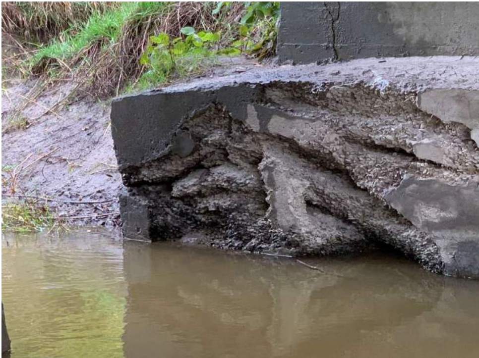
Photo 1-7 - Embankment erosion behind south footing and abutment (Sept. 24, 2020)
