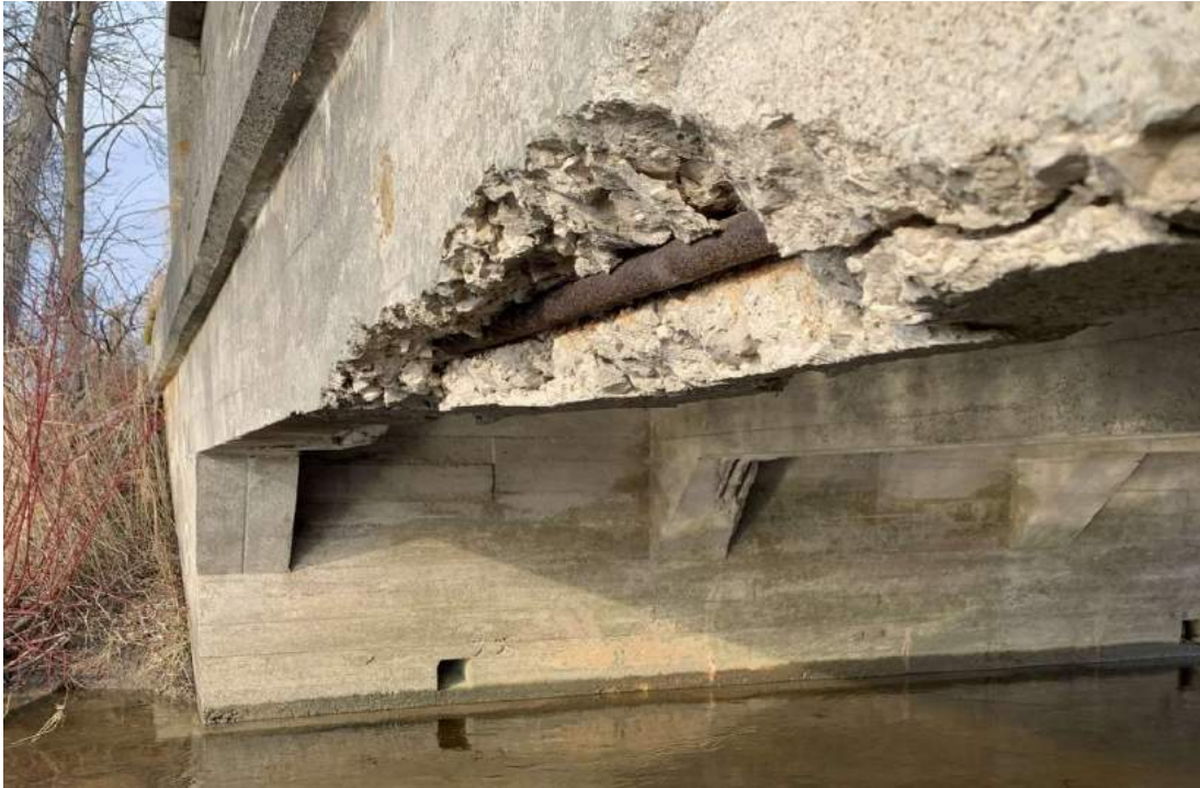
Photo 3-8: Exterior girder delamination and spalling
