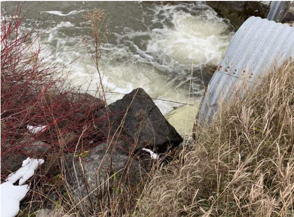
Photo 18-7: Erosion at the haunch of the outlet pipe
