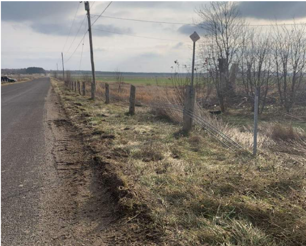
Photo 9-5 - View of 3 cable guiderail barrier protection with loose cable
