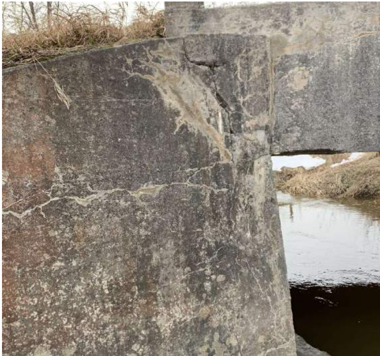
Photo 1-5: Wingwall deterioration (typ)
