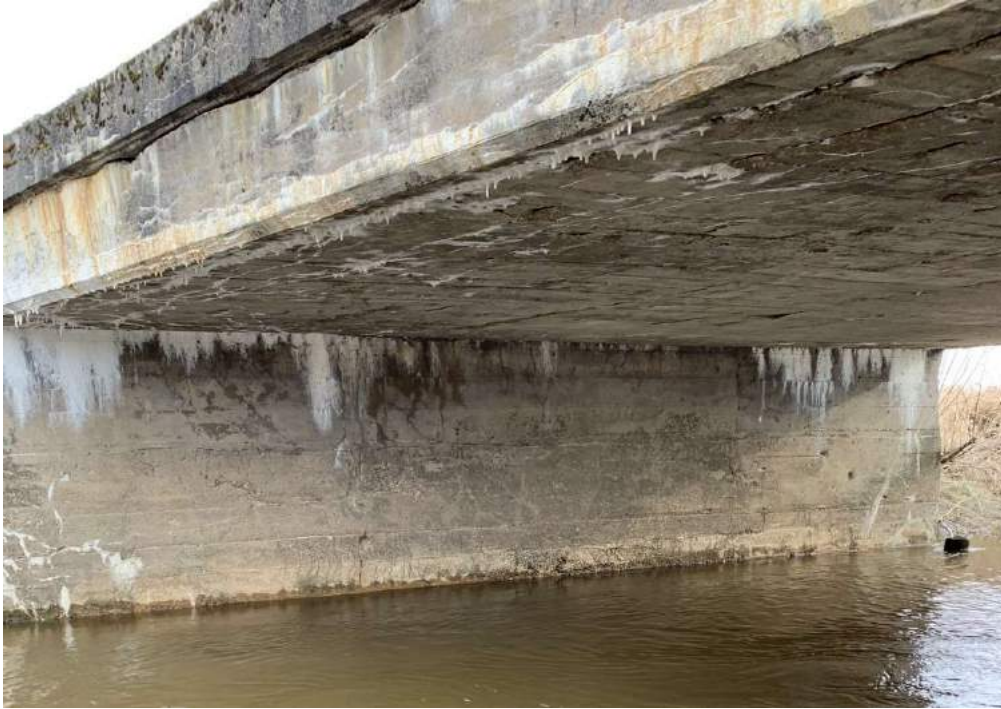
Photo 2-6: Extreme efflorescence at joints
