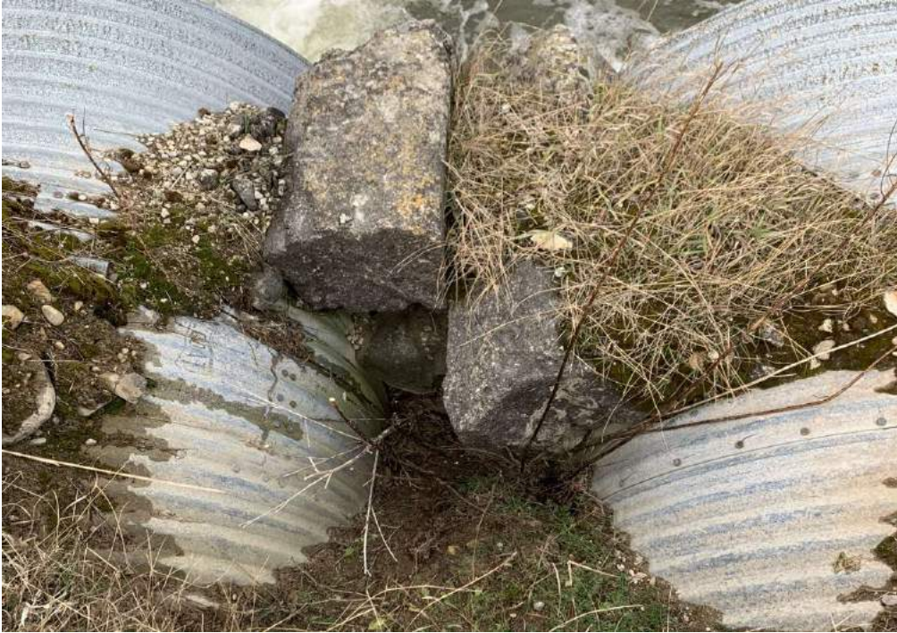
Photo 18-6: View of erosion of embankment and between pipes
