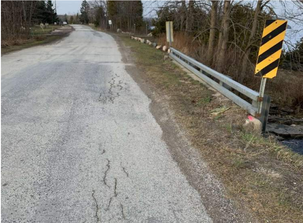
Photo 8-4: Deficient barrier termination and hazard signage
