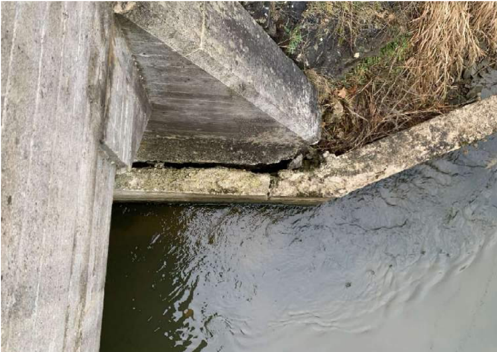
Photo 6-13: Wingwall and footing separation.
