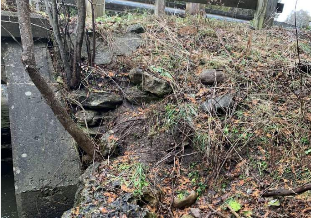
Photo 5-6: Southeast structure embankment erosion
