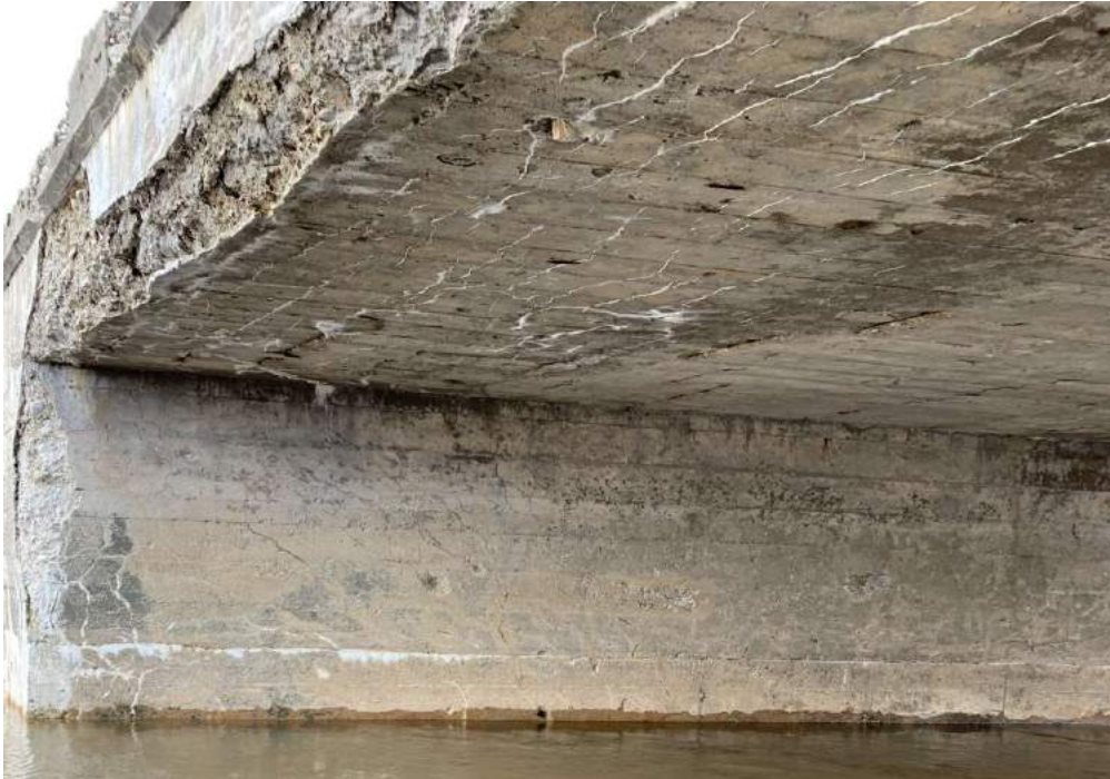
Photo 2-8: Delamination of soffit
