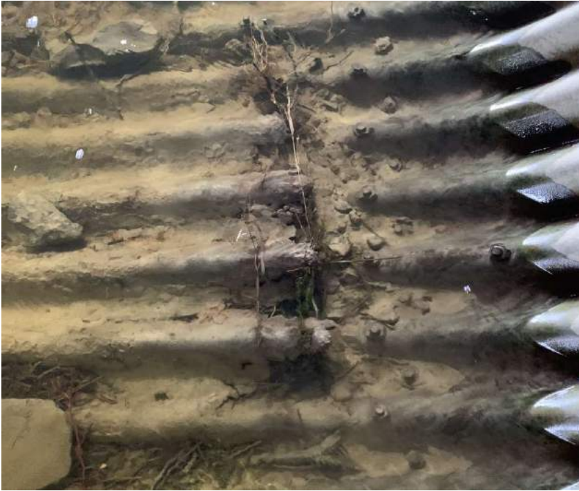
Photo 10-6: Localized failure with complete section loss in base of culvert.
