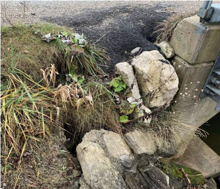
11-5: Rock slope protection and geotextile failure at the southeast quadrant
