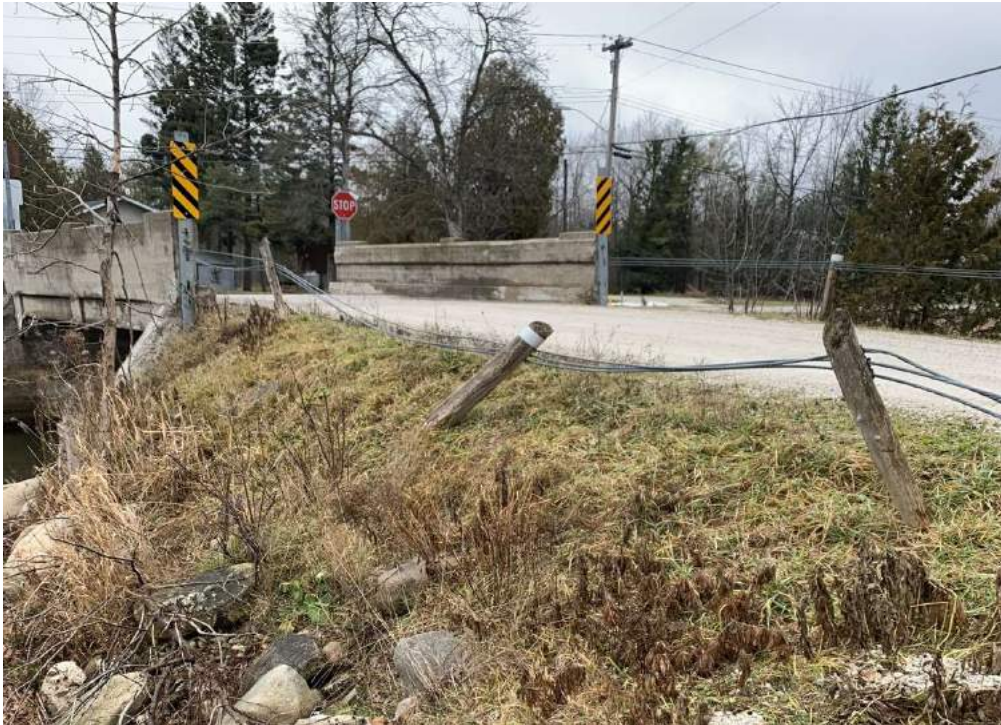
Photo 6-12: Embankment and deficient barrier protection
