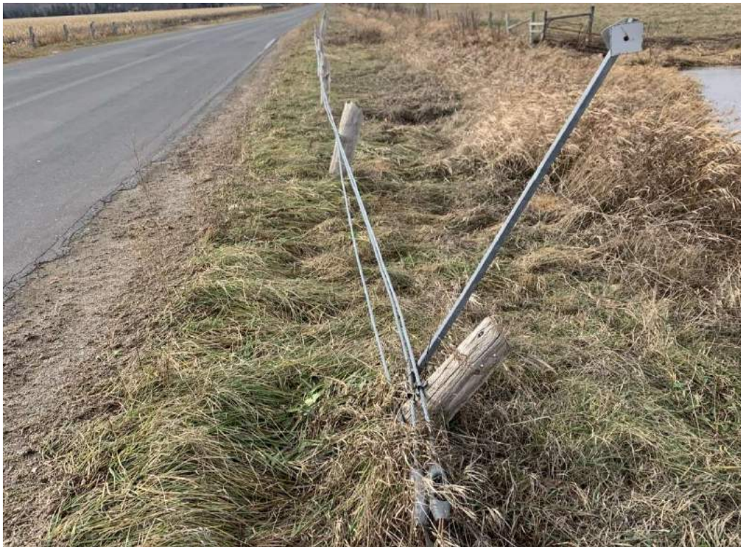
Photo 19-5: Impact damage to the northeast barrier protection post
