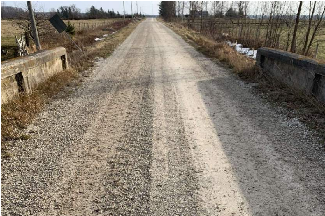
Photo 3-5: Structure and approach wearing surface with wheel path rutting and encroaching vegetation
