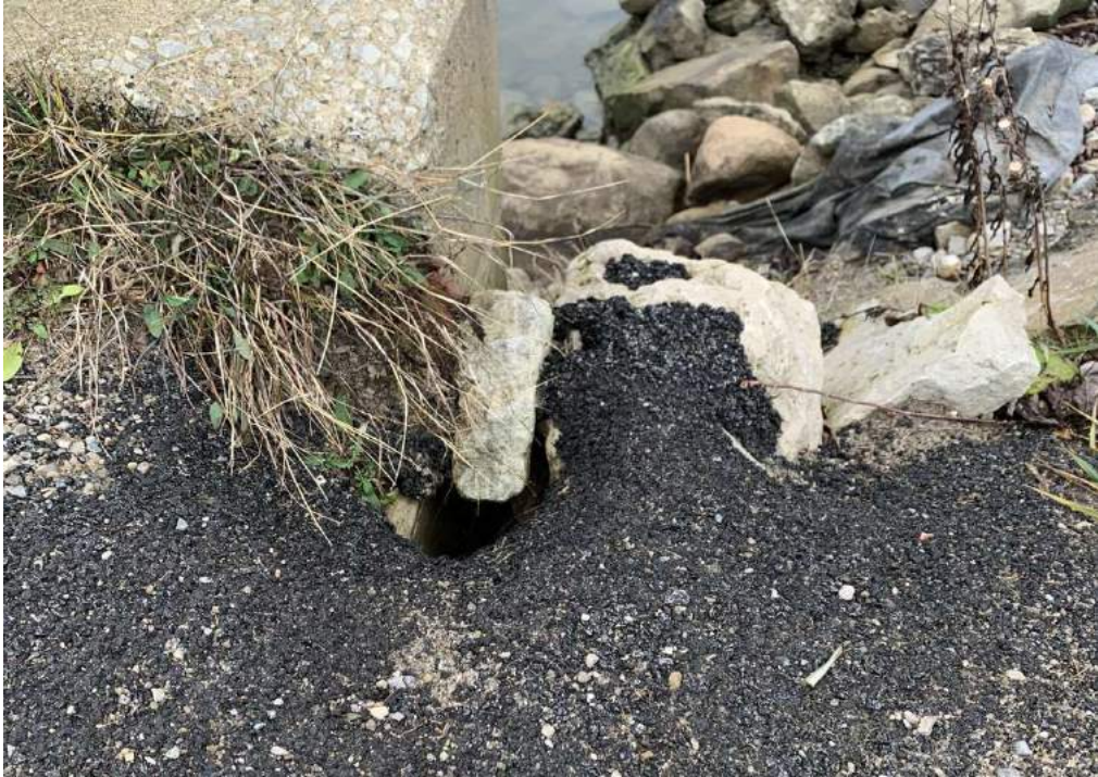
11-10: Minor erosion at the northwest structure quadrant
