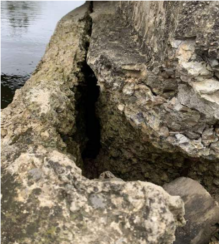
Photo 6-9: Foundation separation and concrete erosion.
