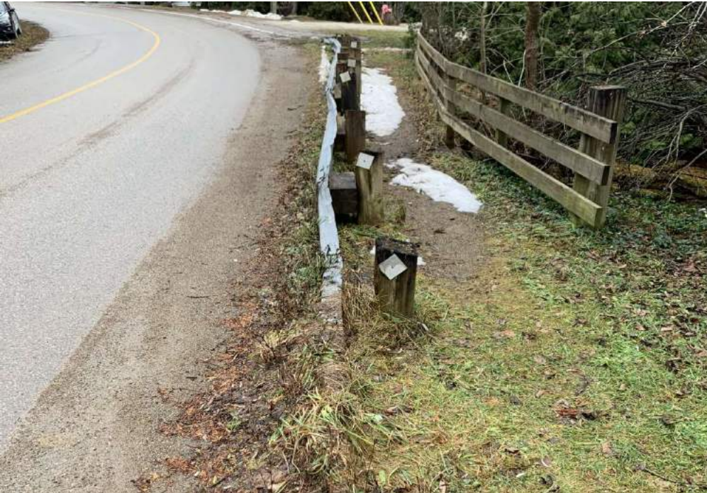
Photo 5-3: Impact damage to southeast barrier protection
