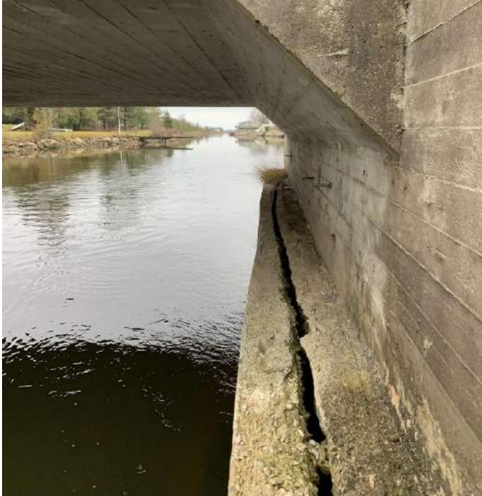
Photo 6-8: View of foundation crack/separation and abutment wall
