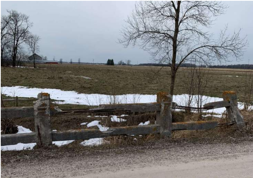
Photo 1-6 - Structure barrier and excessive granular fill on deck
