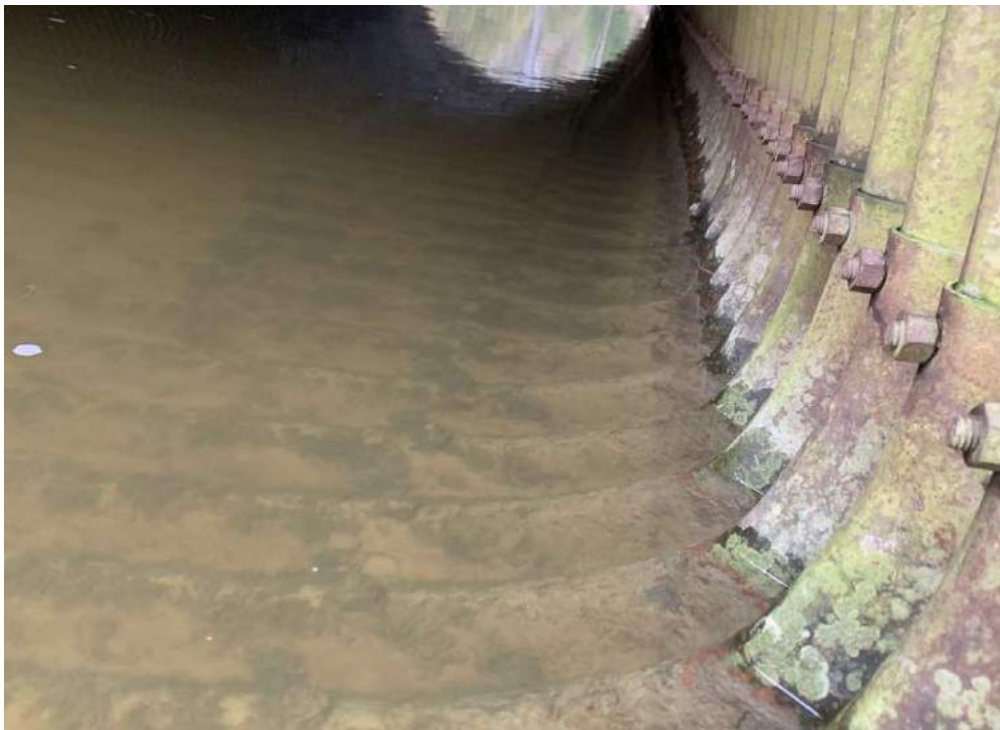
Photo 12-9: View of culvert barrel corrosion at the waterline (typical)
