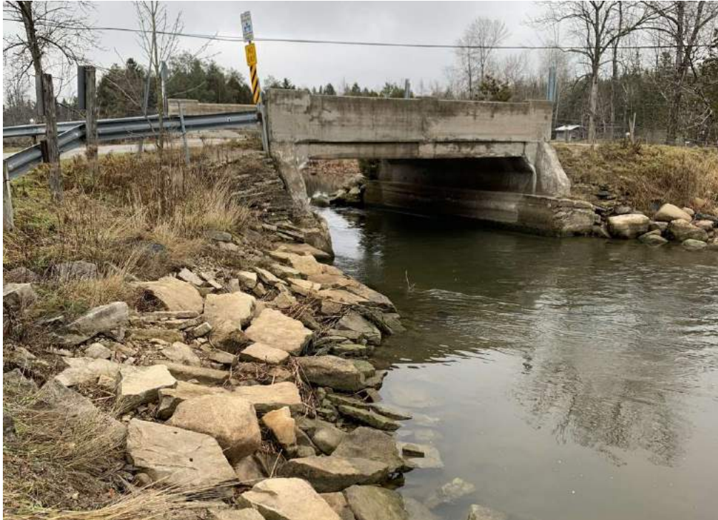
Photo 6-4: View of west structure elevation, slope protection and exterior of parapet wall
