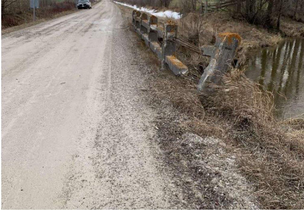
Photo 1-8 - Vegetation and debris accumulation along shoulders, potholes in wearing surface
