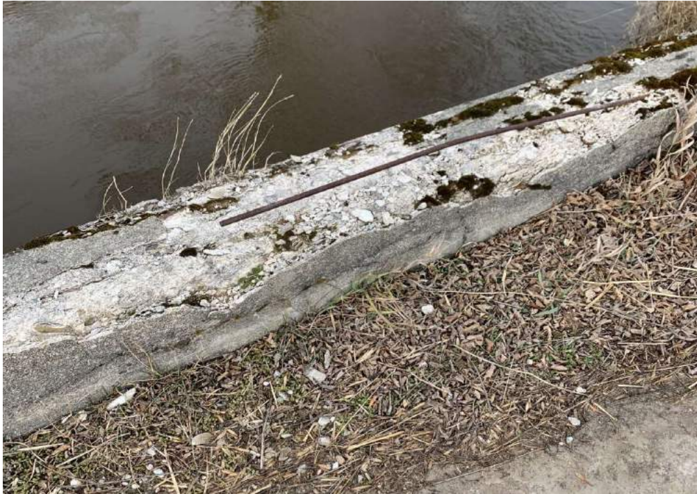
Photo 2-2: Spalling of exterior curb
