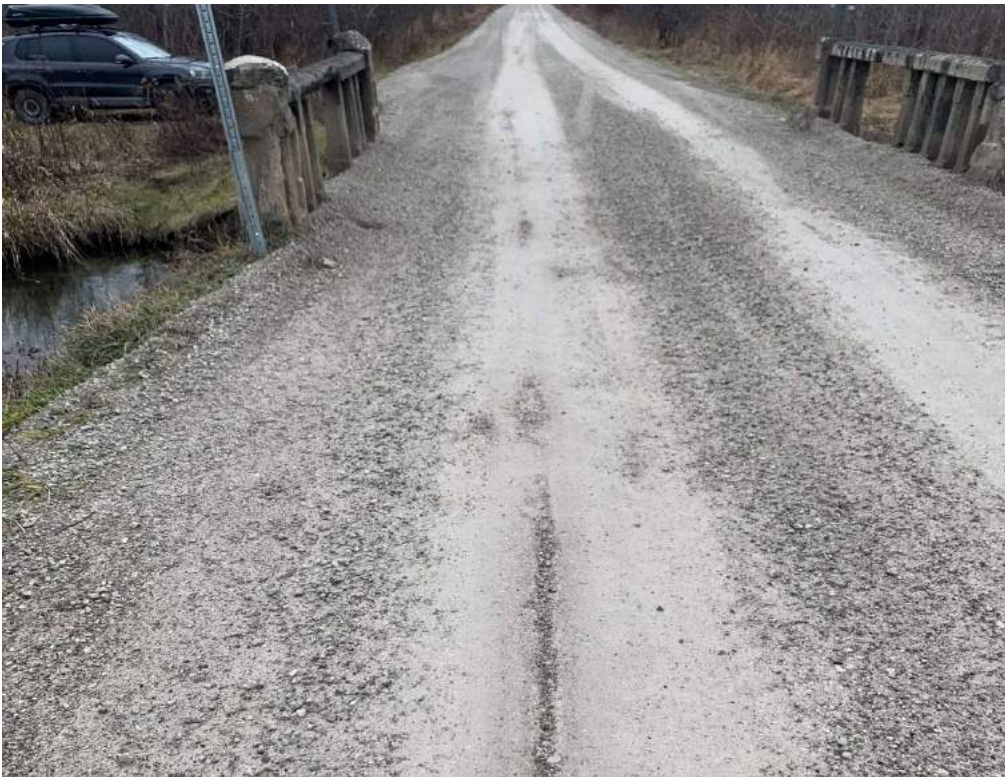
Photo 4-5: Wearing surface deterioration
