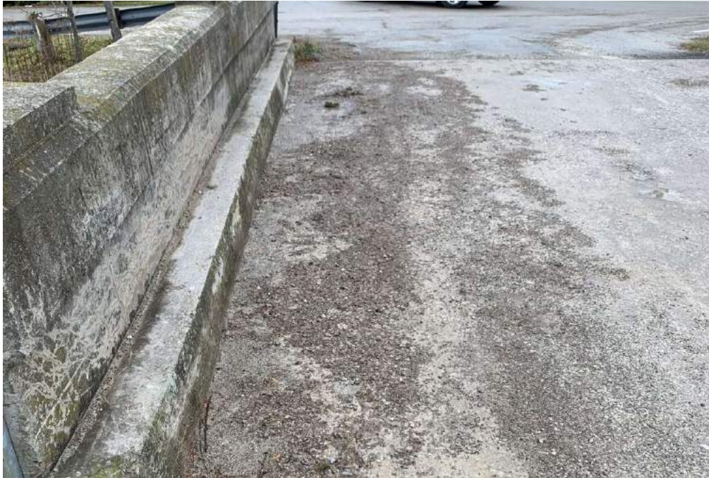
Photo 6-2: View of structure deck with delamination
