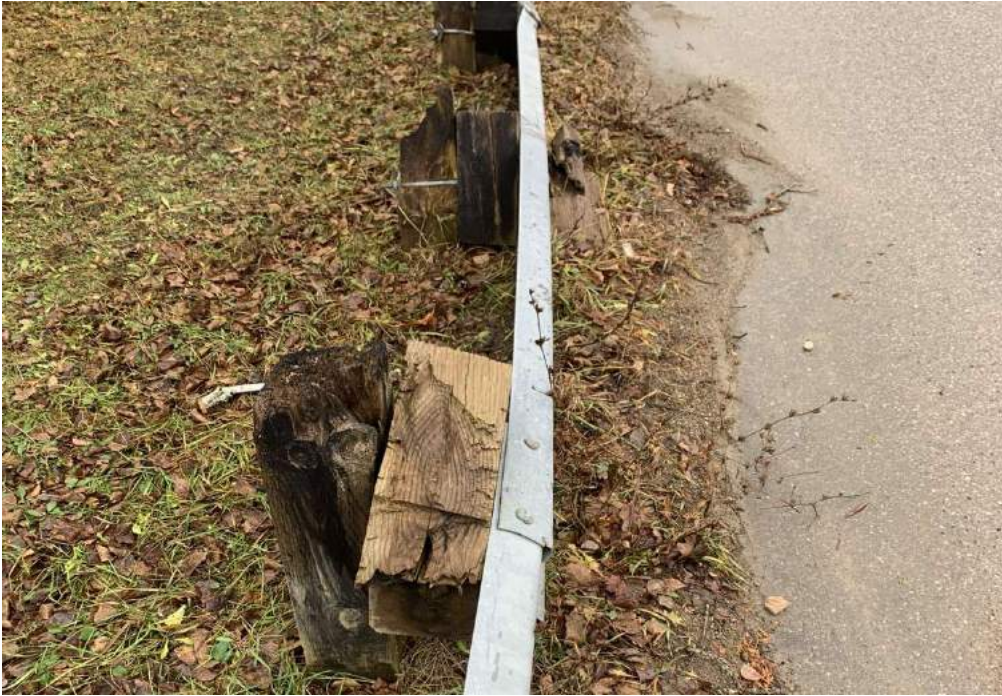
Photo 5-4: Wooden barrier post rot (typical)
