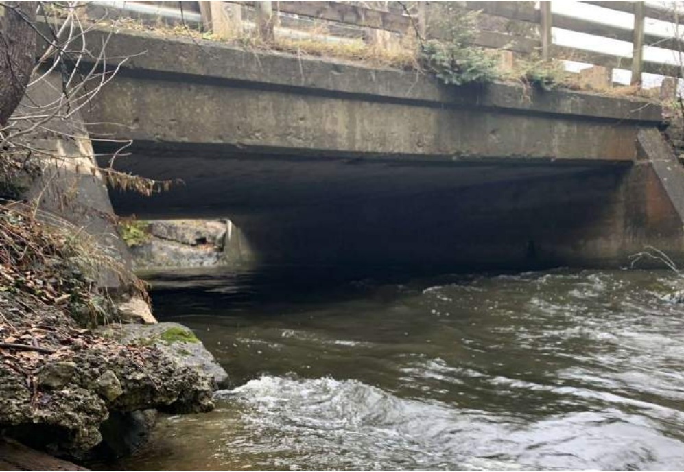
Photo 5-2: View of south structure elevation, exterior curb and soffit, wingwalls and slope protection
