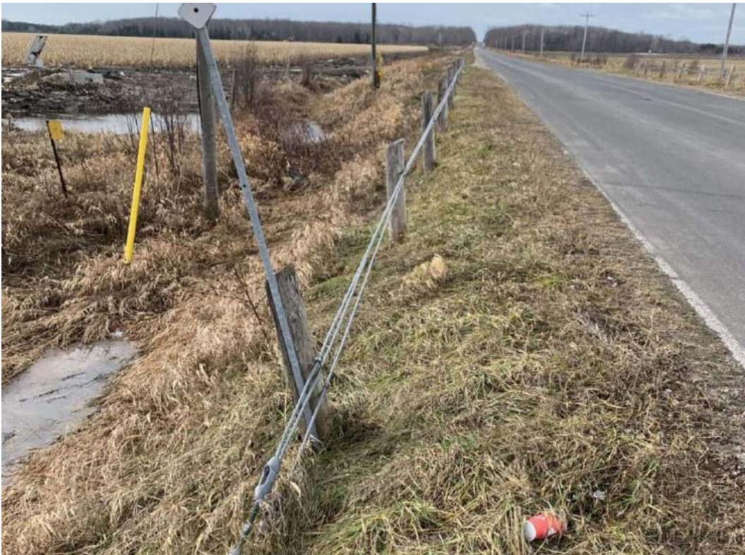
Photo 19-7: View of structure barrier protection (typical)
