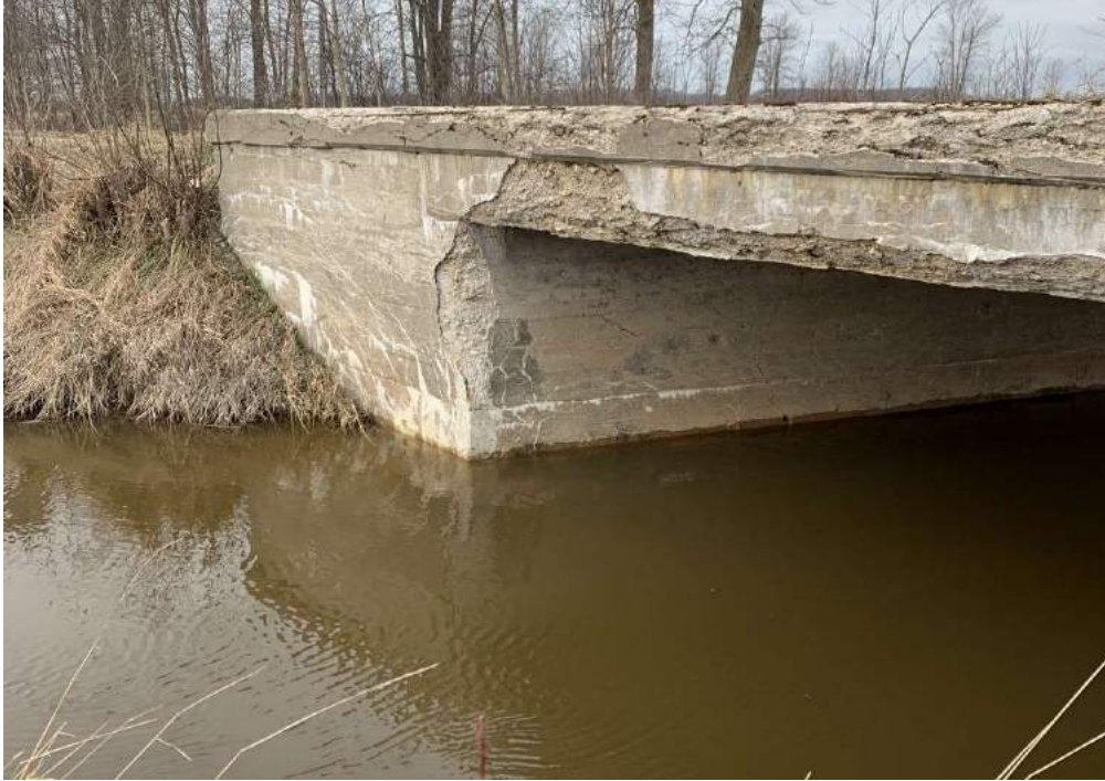
Photo 2-12: Wingwall, abutment wall and exterior soffit delamination.
