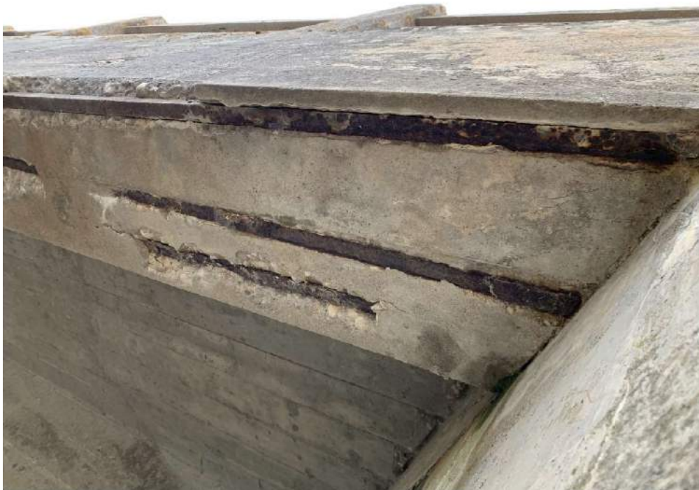
Photo 1-3: North abutment, girders and soffit with spalling and delamination
