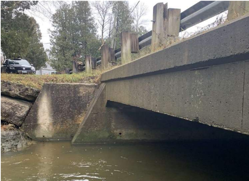
Photo 5-11: View of north structure elevation, exterior curb and soffit and northwest wingwall
