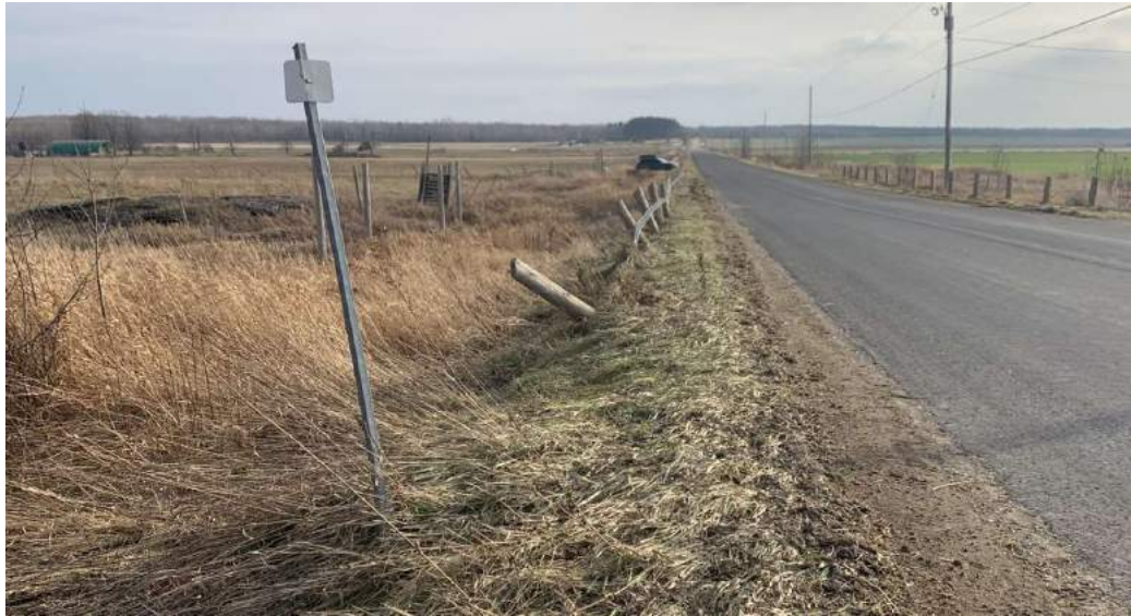
Photo 9-8 - View of northeast deficient section of 3 cable guiderail (impact damage)
