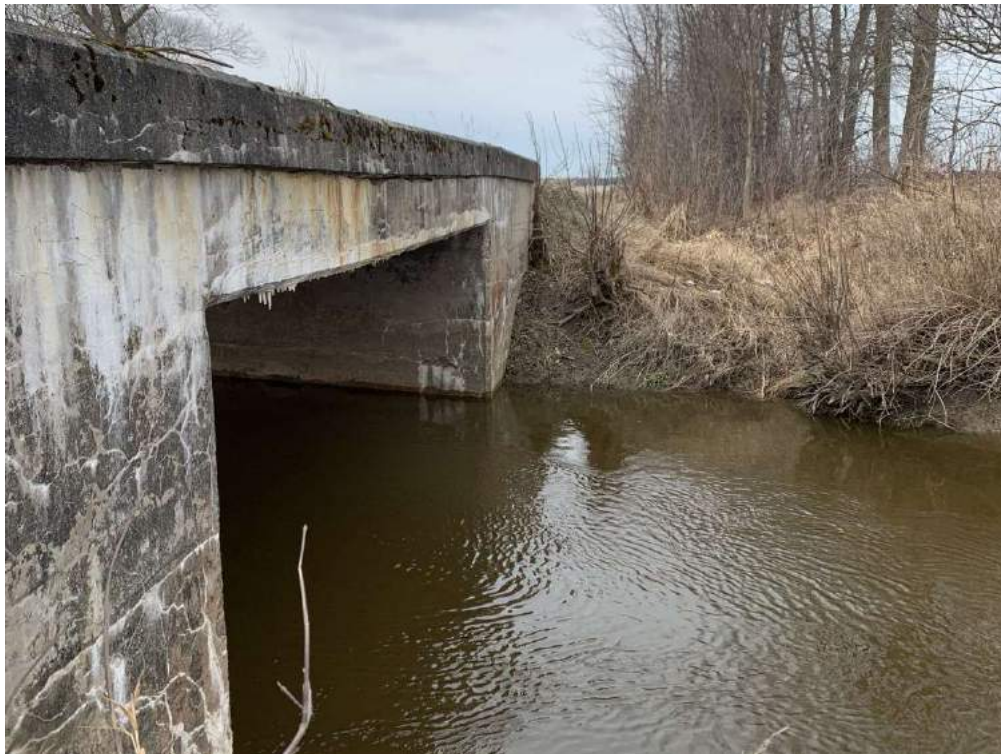
Photo 2-7: Erosion at structure footing, efflorescence of wingwall (typ)
