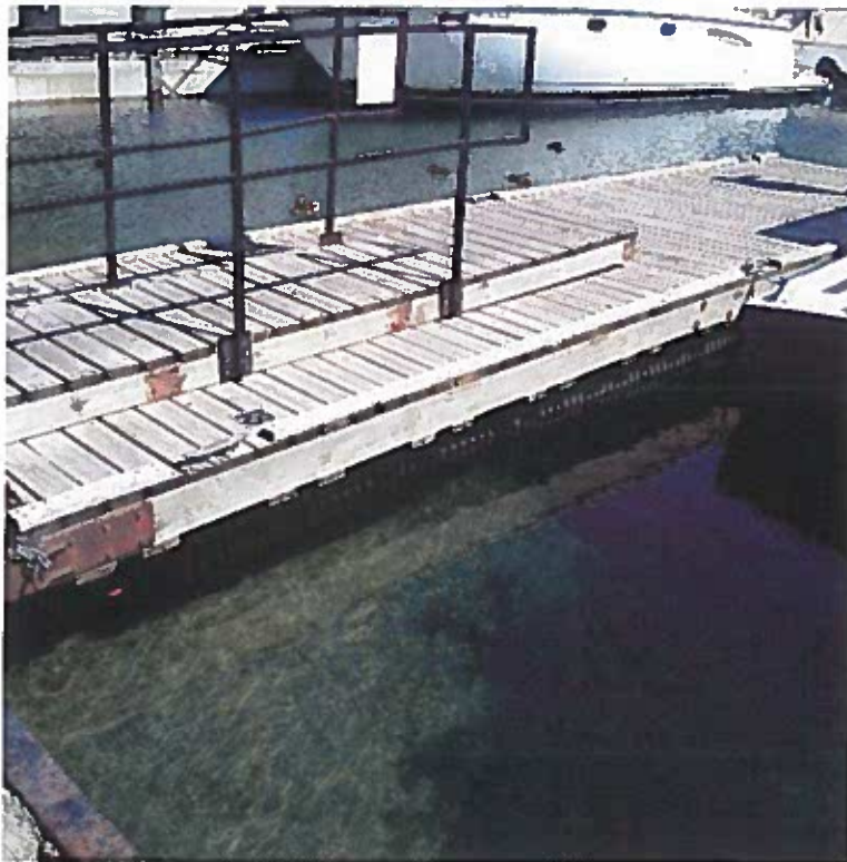
Figure 8: Small Dock to the South of Boat Launch, Looking Northeast from West Wall
