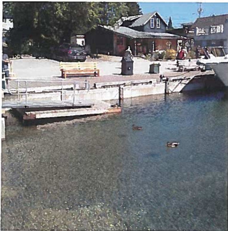
Figure 10: Small Dock to the North of Boat Launch, Looking Northeast from West Wall
